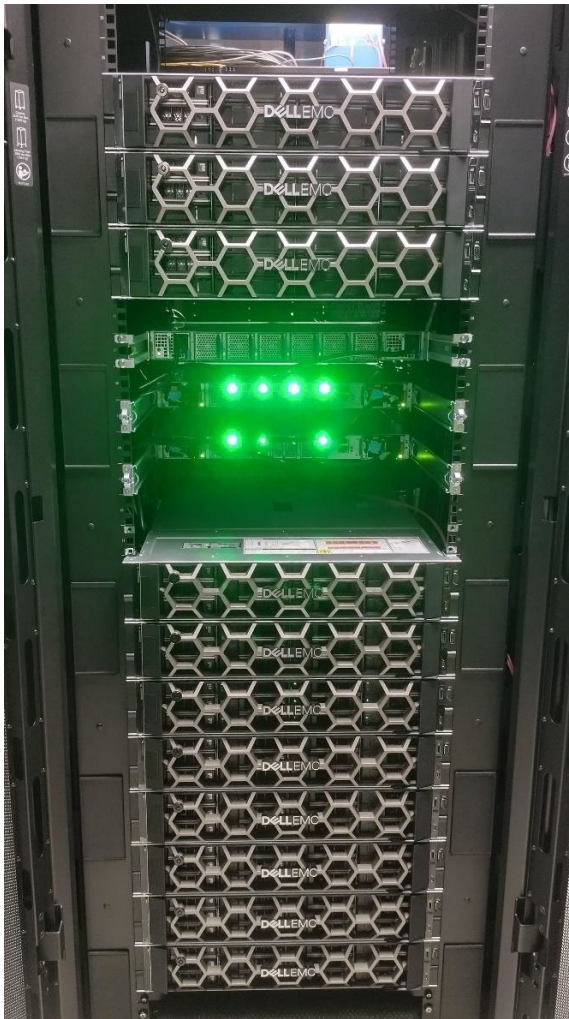
Figure 1: The cluster installed in a single full-scale rack, the master nodes are positioned in the upper part, worker nodes in the lower part.
