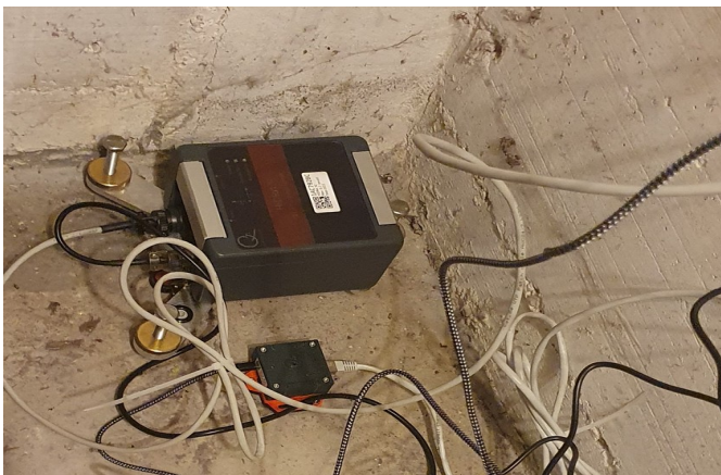
Figure 3: Test installation of colocated MEMS and HiDRA sensor.
